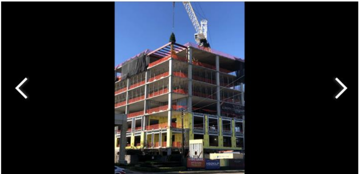
Photo: The Sophie At Bayou Bend
